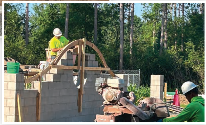
(Right) It's petal to the metal for the English Garden! Construction crews lay the foundation for what will be the backdrop of a beautiful water fountain.
